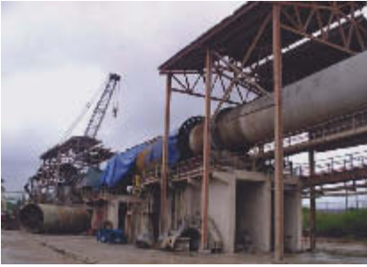
A rotary kiln undergoing maintenance and repair at Omai Bauxite Mining Inc., Guyana. The operation is in the market spotlight owing to it being the only source of refractory grade bauxite outside China, and the subject of a change of ownership to Bosai Minerals of China.
